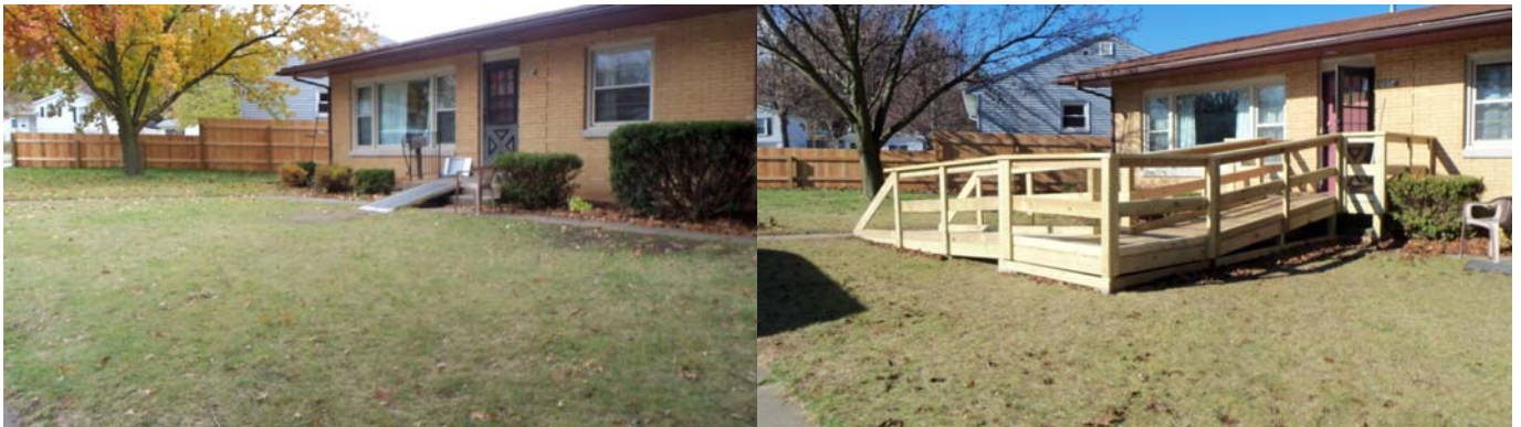
Before and after photos of a home assisted through CDBG with accessibility improvements. With a CDBG grant from the City of Davenport, United Neighbors, a local non-profit organizations, operates the Accessibility Program. The program builds wheelchair ramps, installs grab bars, and makes bathrooms more accessible to low and moderate income residents. The program is free to participants.
