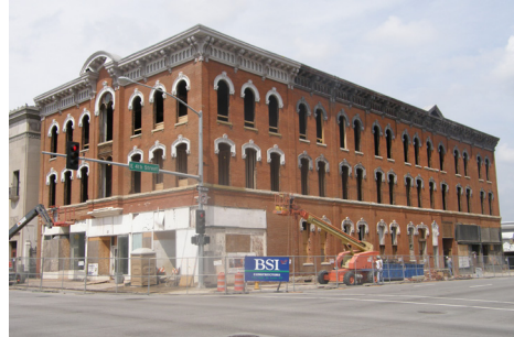
Although this downtown building on 4th Street is now being revitalized, its current state is a legacy of 25 years of urban disinvestment. The City's policies since 2000 have created momentum for investment in downtown, however Davenport's downtown one-way streets remain a disincentive to private investment and are a significant obstacle to restoring the vibrancy of downtown.
